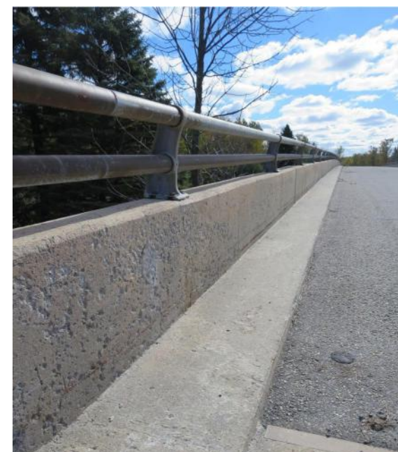
The curb and bridge railing system do not meet current design standards.
