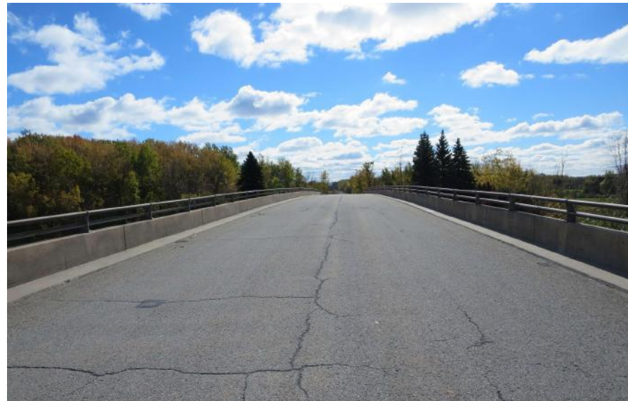
The asphalt wearing surface has wide cracks and raveling throughout.
