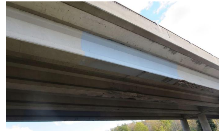
There is concrete deterioration on the underside of the deck and girders. High-load strikes have caused previous damage to the bridge.
