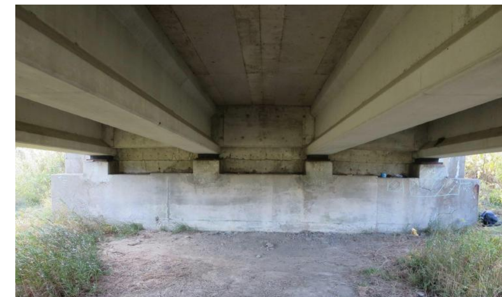
The substructure components are in fair condition with areas of deterioration and cracking.
